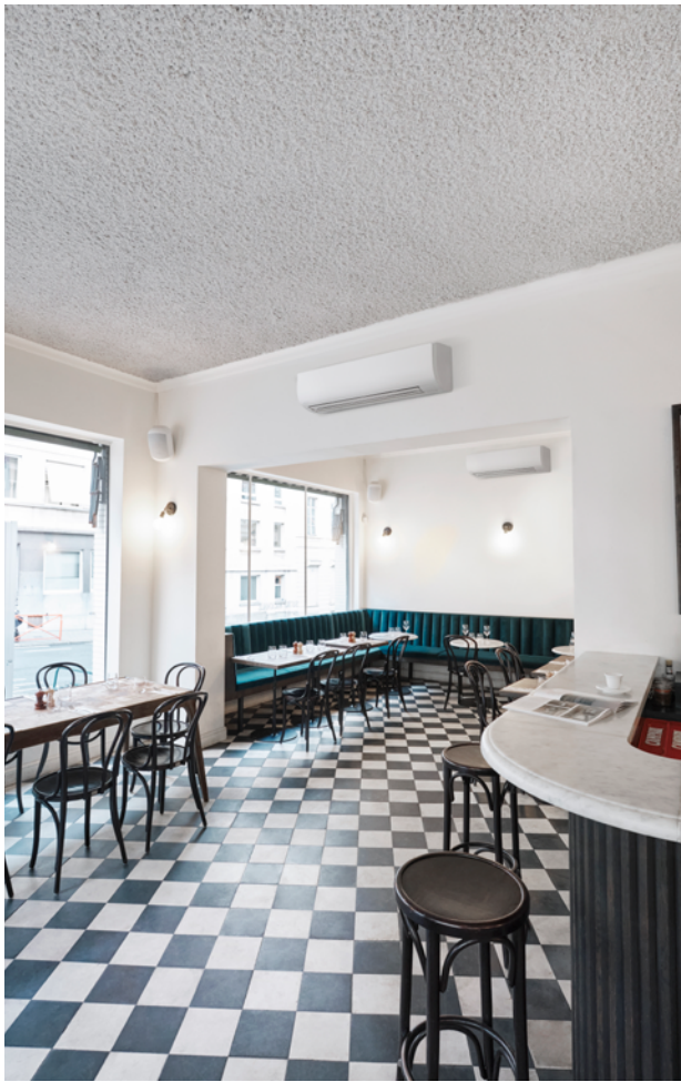
Wall mounted unit
