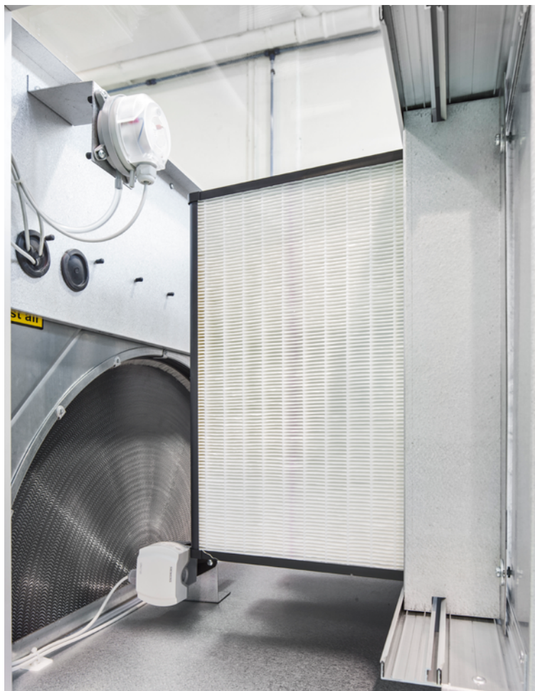
Heat recovery wheel and filter
