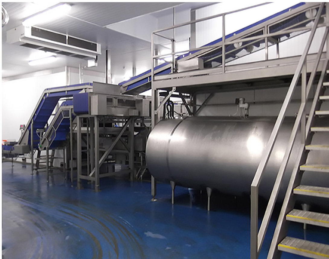
Coombe Fisheries High-performance Zanolli LT refrigeration equipment
